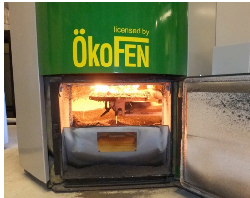
Figure 4. Pellet System Burner
