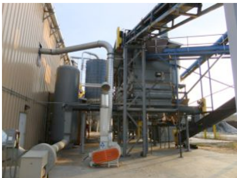
Figure 23. Pellet Processing Equipment
