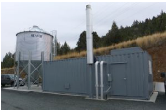
Figure 8. Pellet Silo and Biomass Housing Unit
