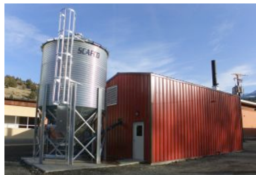
Figure 5. Pellet Silo and Boiler Housing Building
