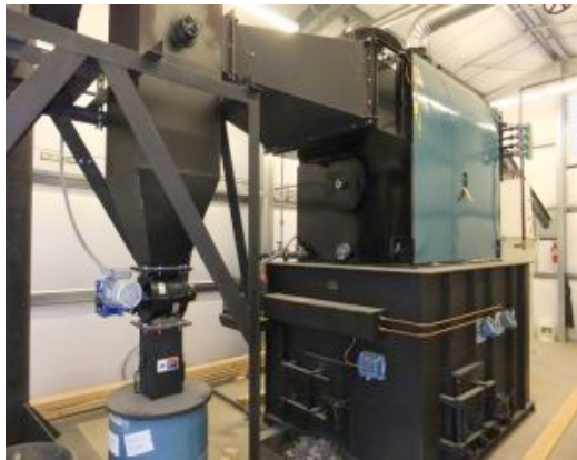
Figure 4. Rear of the Hurst Pellet Unit
