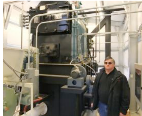
Figure 3. Dennis Flippence, Head of Maintenance, Next to the Pellet Boiler
