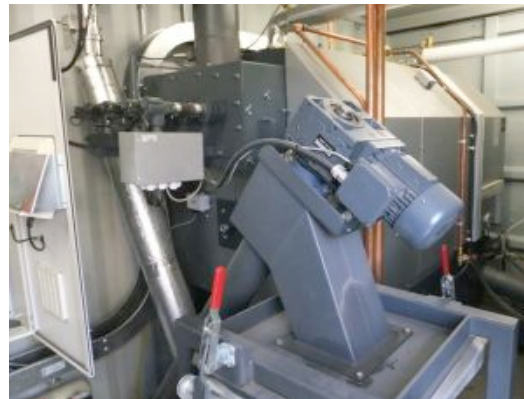
Figure 13. Side View of the Pellet Unit
