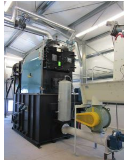
Figure 17. Biomass Combustion Systems Pellet Boiler (photo by Wisewood Inc)
