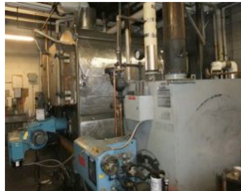
Figure 9. Heating Oil Boiler
