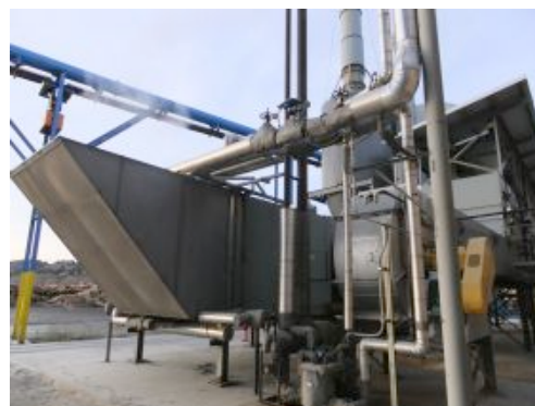
Figure 20. Pellet Drying Equipment
